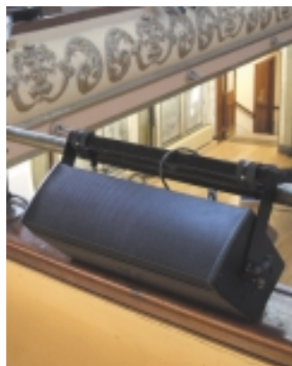
An EM fill located on the balcony
