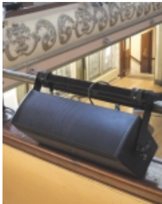
An EM fill located on the balcony
